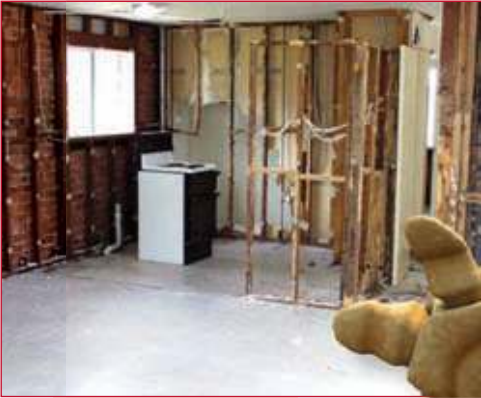
▼ $10,000 damage, not covered by insurance.
