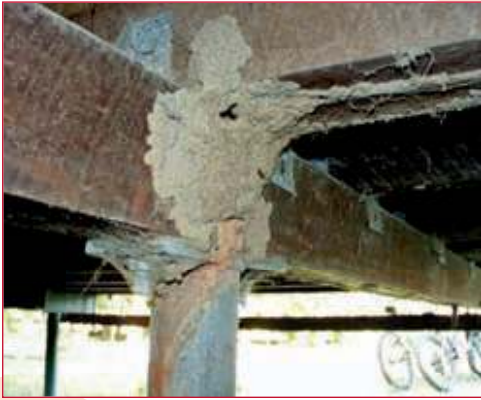
▼ Termites gaining entry into house via steel post.
