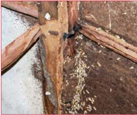
▼ Termites active in wall cavity.
